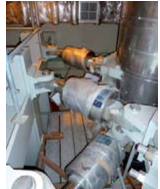
Securing pipe systems with snubbers type 30
